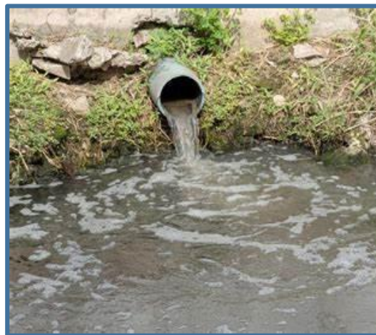
Figure 2. Wastewater from Al-Sharkat Hospital.
