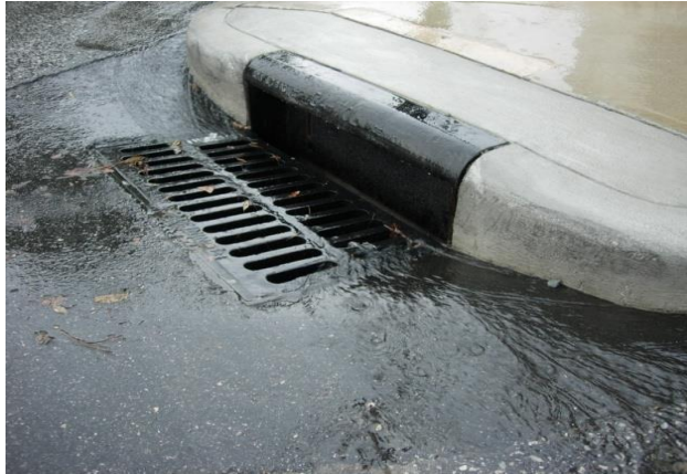
Figure 4: Modern drainage system.
