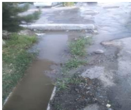
Figure 3: violation of the operation of the water drainage system
