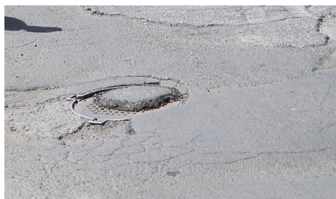
Engineering communication wells located in the traffic section
